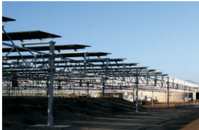
Greenhouse solar collection array
