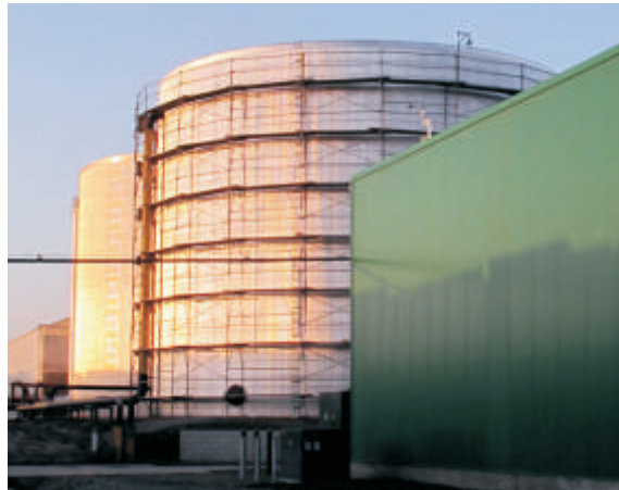
Thermal storage tanks
