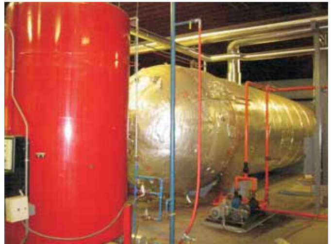
Insulated Heat Storage Tank
