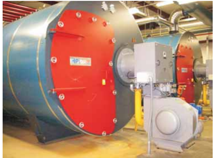
High Mass Boilers
